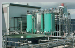
Avlon Wastewater Treatment Plant /22
